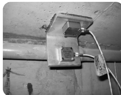
Corrosion sensor embedded in a concrete structure
